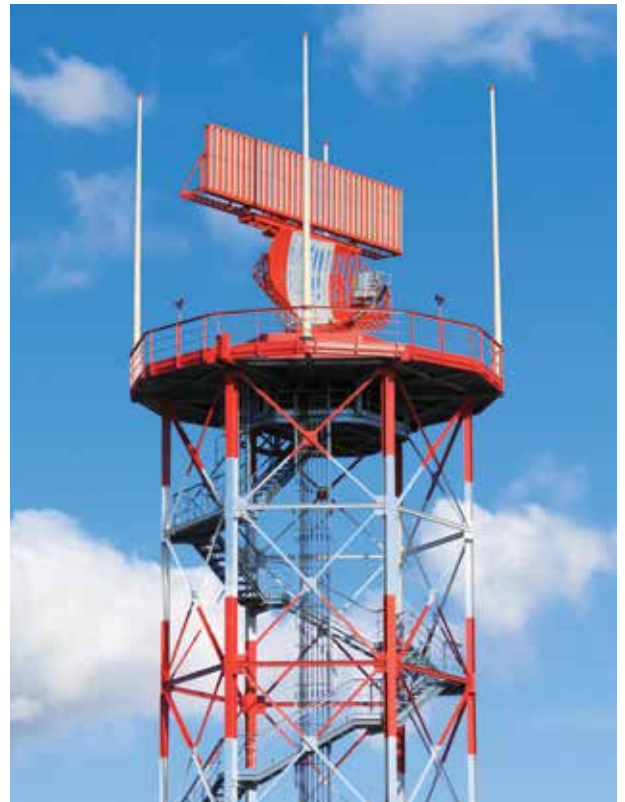
Co-mounted MSSR and passive ADS-B system
